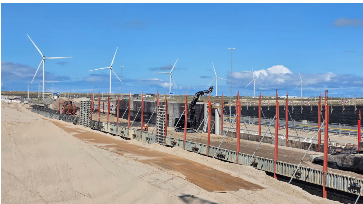
Building of earth retaining structure on the side with the Maasvlakte beach
